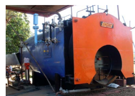
6 TPH 'D' Type Boiler
