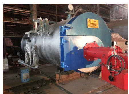
4TPH Oil Fired Boiler
