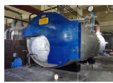
Solid Fuel Boiler
