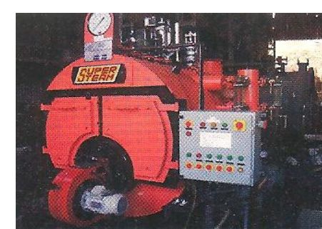
Coal Fire Boiler
