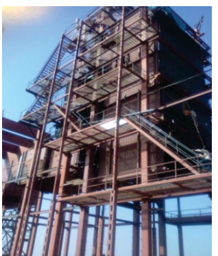
Boiler Side View
