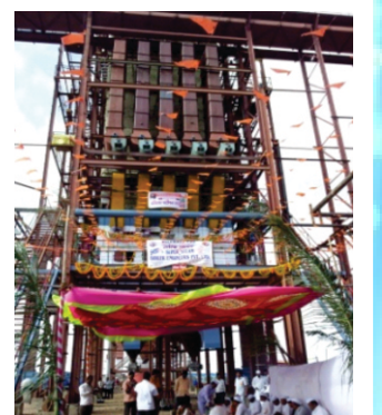
Boiler Front View
